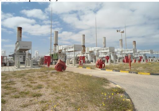
Figure 1: Sirte Oil & Gas Co Natural Gas Station of at Marsa El-Braga [1].
