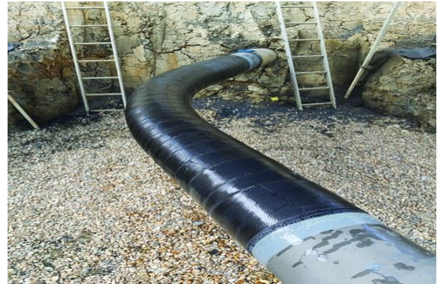
Figure 12- Applied to a pipeline bend [3].
