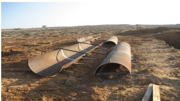
Figure 5: 36 inch Fabricated Split Pipe Sleeve- [1].
