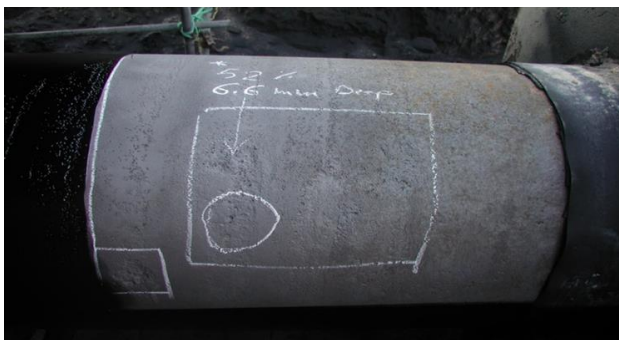
Figure 4- Pitting Corrosion, Defect Location determined by Rosen Smart Pig [1] [2]
