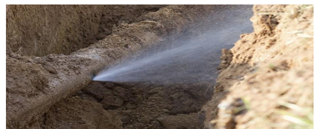
Figure 7: Pipe section leak caused by Stress Corrosion Cracking [1].
