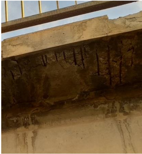
Figure 9. Reinforcement steel rust
