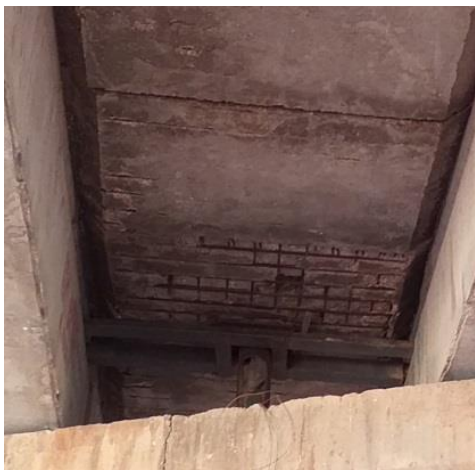
Figure 10. Collapse of concrete cover
