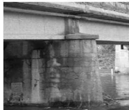
Figure 1. Cracking in bridge due to sulfate attack
