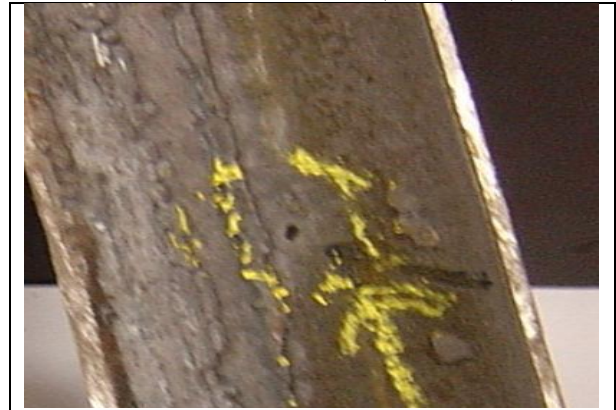
Figure 2a. Caustic Gouging
