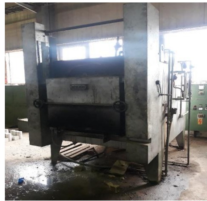
Figure 2 Electric furnace used
